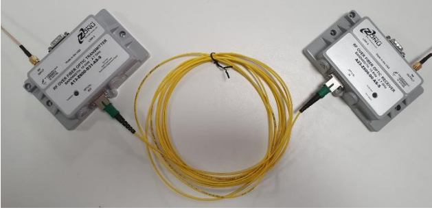
Fig. 2. OZ600 modules connected with an optical fiber. Coaxial cables used for transferring radio signal can also be seen on the sides.
